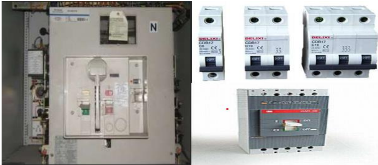
Figure 8: Different types of circuit breaker used in Santahar.
