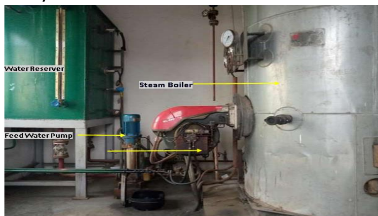
Figure 2: Start-up Boiler/ Auxiliary Boiler
