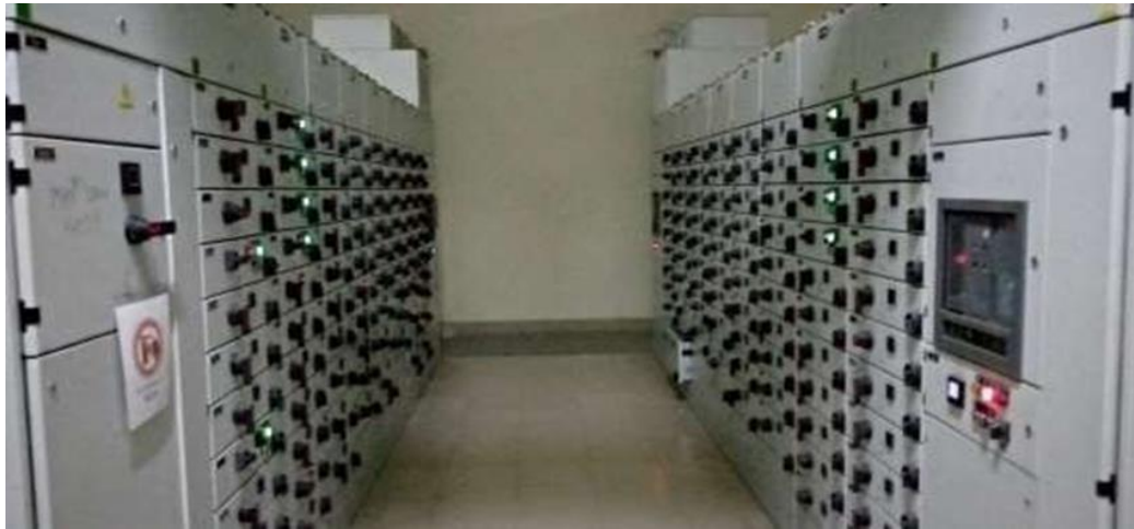
Figure 5: M.V switchgear room
